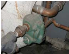
Typical steam trap installation
