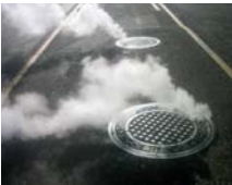
A leaking steam trap
